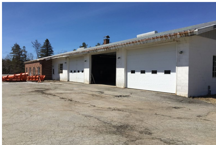
Photo-2: Rear right side view of existing building. Siding and building trim in need of replacement. Note holes in roof trim where pigeons and animals have access to building interior. Also, end of roof is too low for building extension to increase storage or headroom inside the building.
