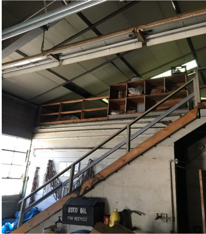
Photo-7: View of interior of building. Note uninsulated ceiling panels.
