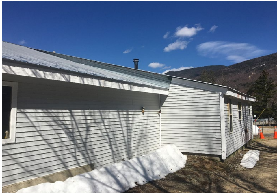
Photo-2: Rear view of existing patrol shed. Siding and building trim in need of replacement. Also, shed end of roof is too low for building extension to increase storage or headroom inside the building. The work room addition on the back provides space for the snowplow when 10-wheeler is parked inside.
