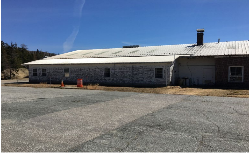
Photo-5: View of left side of existing building. Note rotten siding, deteriorated roof and holes in roof trim allowing access by pigeons and animals.
