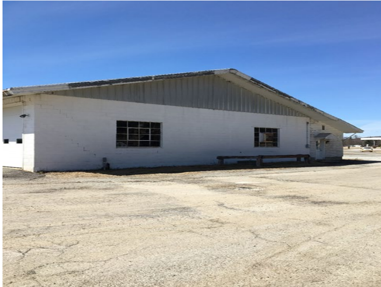
Photo-1: Rear view of existing building. Note deteriorated condition, single pane windows, rotten trim and cracks in uninsulated cinder block walls.
